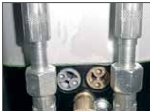
By pass valves
